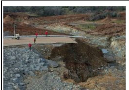
California Department of Water Resources crews inspect and evaluate the erosion just below the Lake Oroville emergency spillway site after lake levels receded on February 13.
