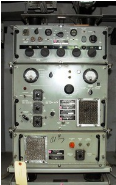
One of the Battleship Iowa 's AN/URT-23(C) transmitters. The exciter is at the top, the PA is in the middle, and the amplifier power supply is on the bottom. [Jim Jerzycke, KQ6EA, photo]
