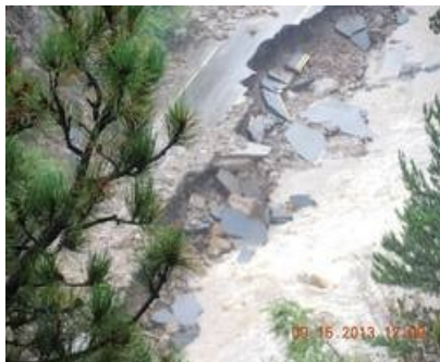
A road washout in Left Hand Valley [Boulder County photo]
