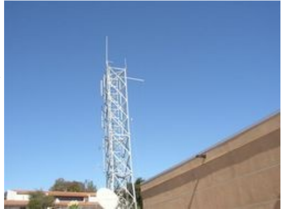
The tower at the Santa Barbara County EOC, with tri-band antenna on the left and HF antenna on the cross arm on the right. The third rod is the lightning rod. (photo courtesy N6ZKJ)
